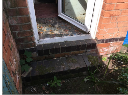
Photo - 23 Cracking beneath back door on rear elevation
