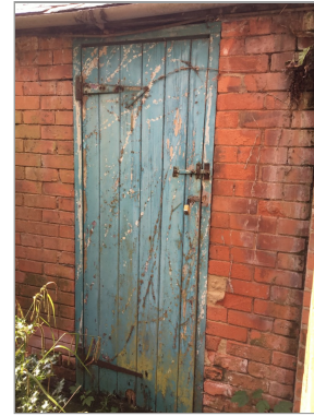
Photo - 99 Door and frame in poor condition
