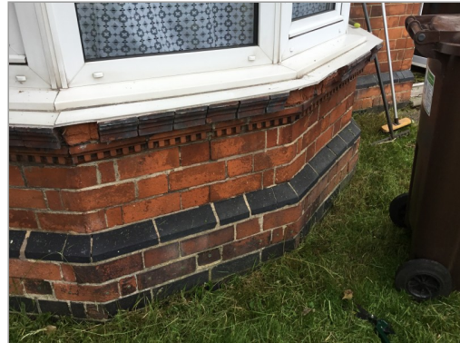
Photo - 15 Damaged bricks beneath front bay. Also note injected DPC
