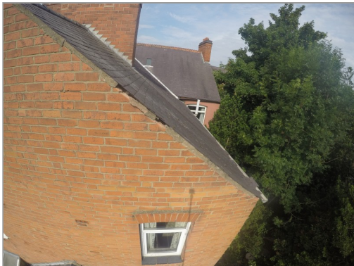
Photo - 9 Loose verge pointing
