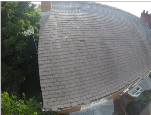
Photo - 5 Front pitch with numerous slipped slates.
