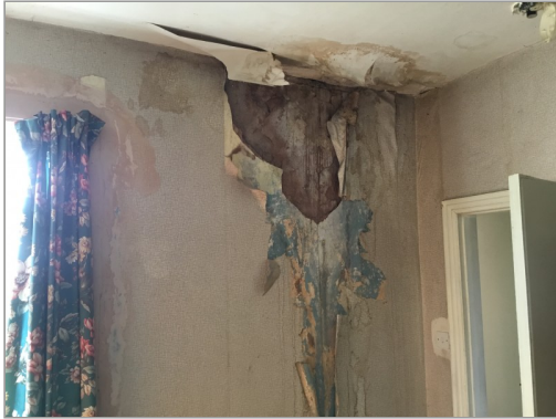
Photo - 60 Damaged middle bedroom due to leak in roof
