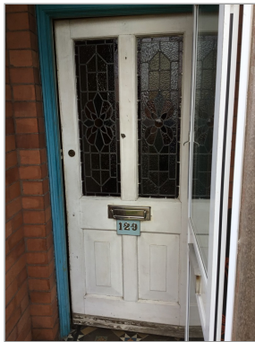
Photo - 80 Inner front door of dated design with no safety glass
