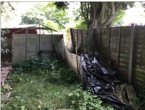
Photo - 108 Fences in poor condition
