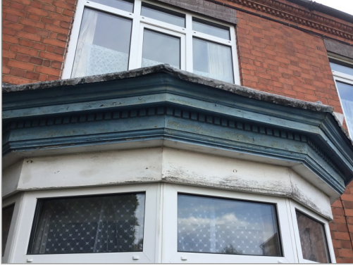
Photo - 33 Fascias in poor decorative condition
