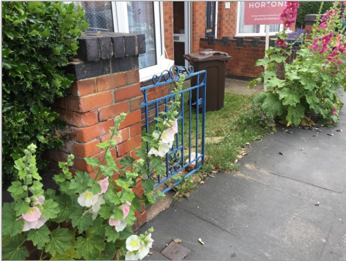
Photo - 106 Boundary wall in poor condition with sections missing
