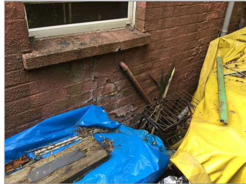
Photo - 19 Textured coating in poor condition
