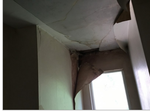
Photo - 48 Landing ceiling at junction with rear projection
