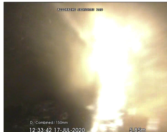
Photo: 4_8A, 00:00:41 5.68m, Joint displaced, medium (between 1.0 and 1.5 times the pipe wall thickness)
