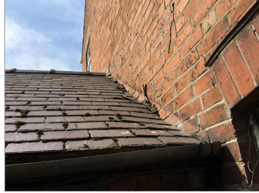
Photo - 97 Lead flashing required
