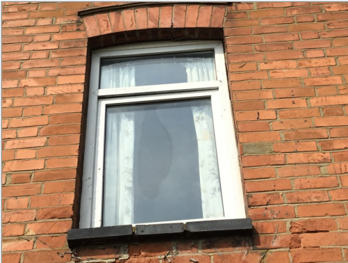
Photo - 26 Blown seals
