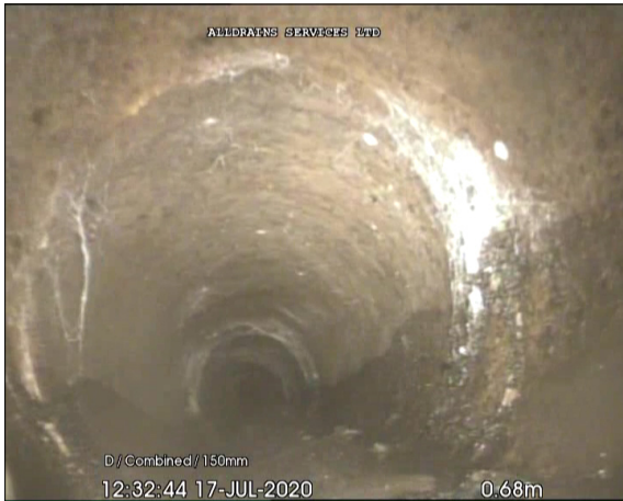
Photo: 4_4A, 00:00:10 0.68m, Joint displaced, medium (between 1.0 and 1.5 times the pipe wall thickness)
