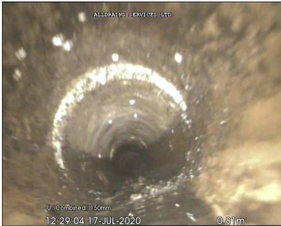
Photo: 2_4A, 00:00:09 0.91m, Joint displaced, medium (between 1.0 and 1.5 times the pipe wall thickness)
