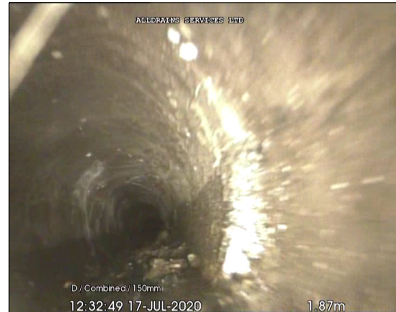
Photo: 4_5A, 00:00:14 1.87m, Joint displaced, medium (between 1.0 and 1.5 times the pipe wall thickness)
