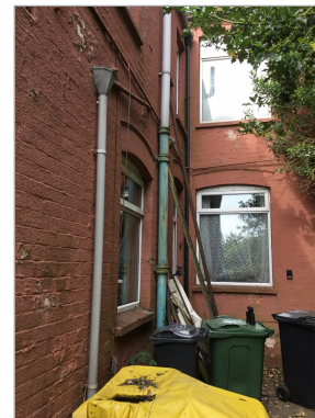
Photo - 94 Lower cast iron soil and vent pipe in poor condition
