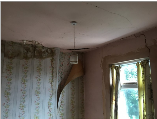
Photo - 58 Damage in back bedroom most likely due to roof leak and also cracking on rear elevation (see section E4)
