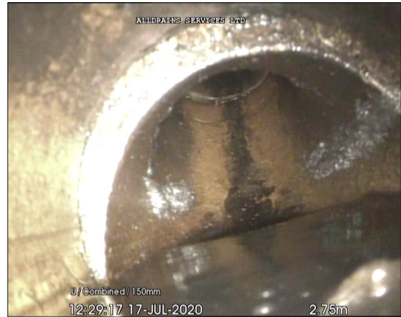
Photo: 2_5A, 00:00:22 2.75m, Joint displaced, medium (between 1.0 and 1.5 times the pipe wall thickness)
