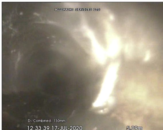
Photo: 4_6A, 00:00:39 5.09m, Joint displaced, medium (between 1.0 and 1.5 times the pipe wall thickness)
