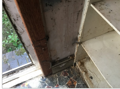
Photo - 67 Crumbling plaster and high moisture content in kitchen by door
