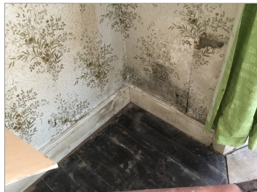
Photo - 65 High moisture content and crumbling plaster in front reception
