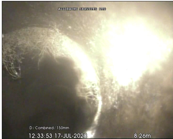
Photo: 4_9A, 00:00:52 8.26m, Roots, fine at joint
