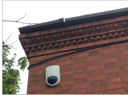
Photo - 13 Loose bricks beneath disconnected gutter in front left corner.
