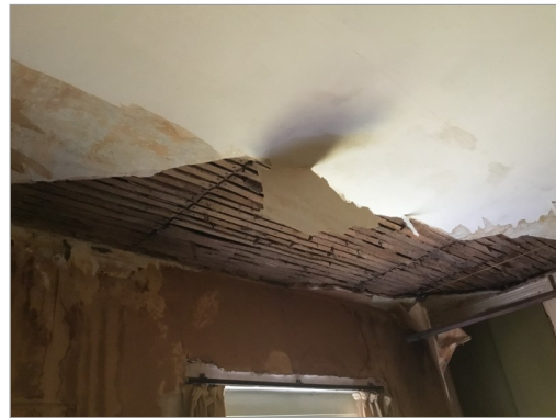
Photo - 44 Damaged ceiling in rear reception
