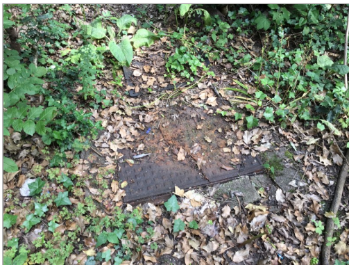
Photo - 93 Unable lift lid as it is broken
