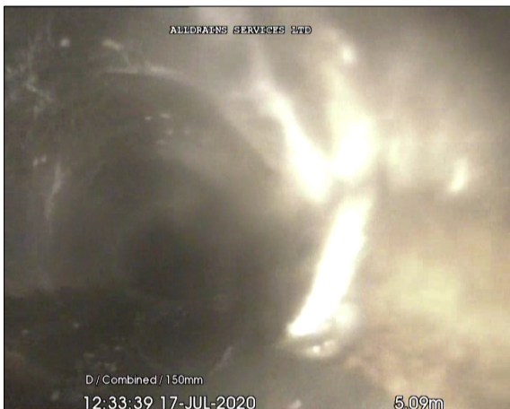
Photo: 4_6A, 00:00:39 5.09m, Joint displaced, medium (between 1.0 and 1.5 times the pipe wall thickness)
