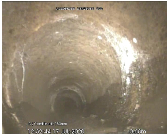
Photo: 4_4A, 00:00:10 0.68m, Joint displaced, medium (between 1.0 and 1.5 times the pipe wall thickness)
