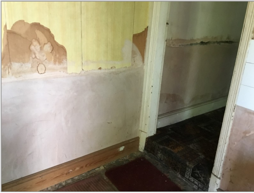
Photo - 68 High moisture content in party wall despite it being a newer plaster. Note "tide mark" in rear reception
