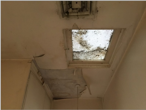
Photo - 49 Damage around loft hatch on landing
