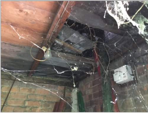
Photo - 98 Unable to enter loft area due to stored items
