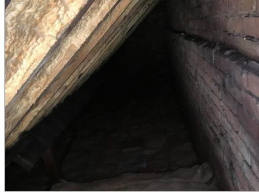
Photo - 40 Unable to enter rear projection loft area
