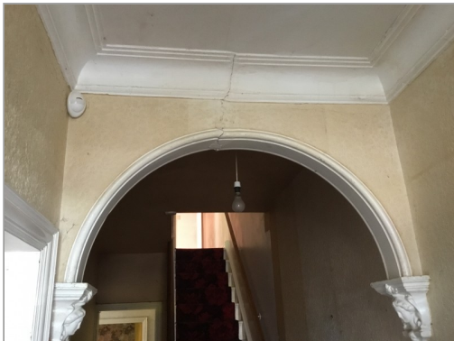
Photo - 52 Cracking in hallway
