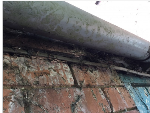
Photo - 103 Wallplate rotten and contains wood boring beetles
