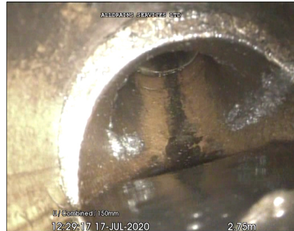
Photo: 2_5A, 00:00:22 2.75m, Joint displaced, medium (between 1.0 and 1.5 times the pipe wall thickness)
