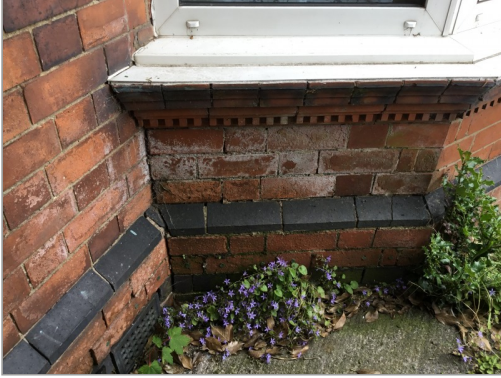
Photo - 16 Spalled bricks and weathered mortar
