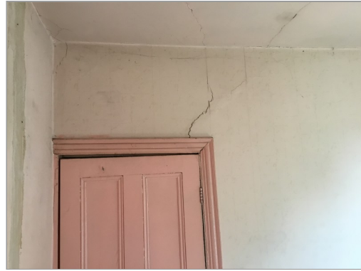
Photo - 57 Distortion in back bedroom door frame suggests historic movement toward the left elevation has occurred.
