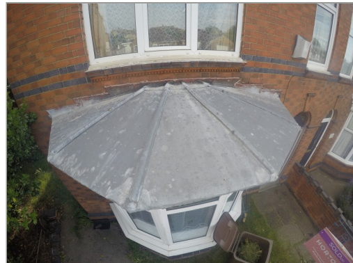
Photo - 10 Bay roof. Note loose flashings. This might explain water staining to ceiling in front reception
