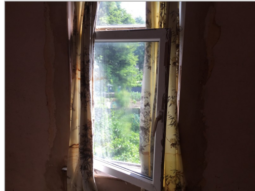
Photo - 27 Handle and lock broken on fire escape window in back bedroom
