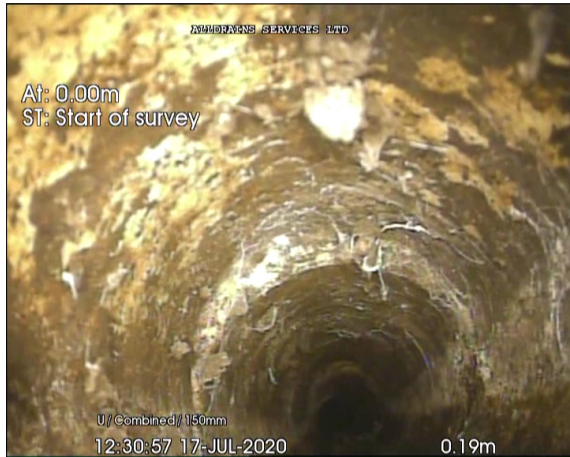
Photo: 3_4A, 00:00:07 0.18m, Joint displaced, medium (between 1.0 and 1.5 times the pipe wall thickness)
