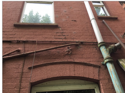
Photo - 21 Cracking apparent over rear projection
