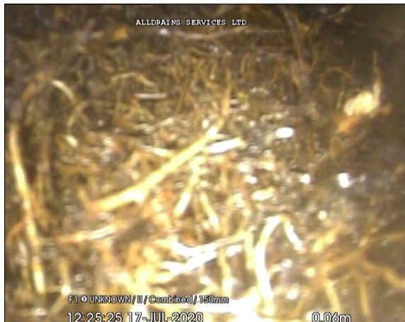
Photo: 1_4A, 00:00:11 0.6m, Roots, mass, 95% cross-sectional area loss
