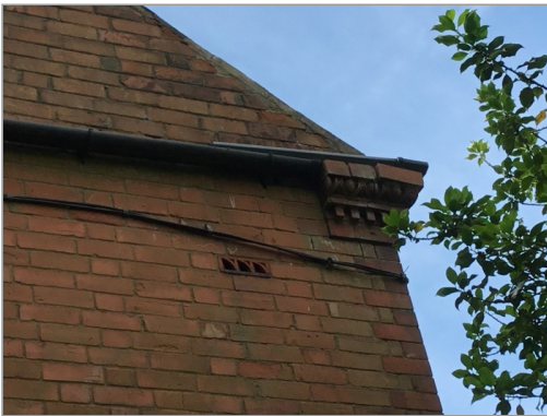
Photo - 11 Poor connections
