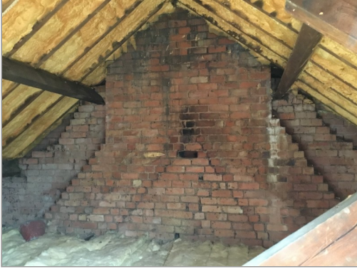
Photo - 1 Chimney in right gable. Sections of gable appear to only be single skin thickness
