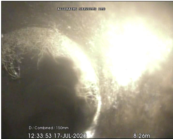
Photo: 4_9A, 00:00:52 8.26m, Roots, fine at joint
