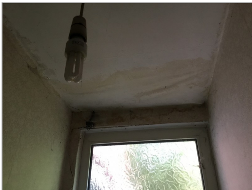
Photo - 45 Water staining over side door
