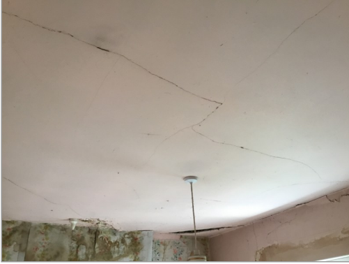
Photo - 47 Back bedroom ceiling
