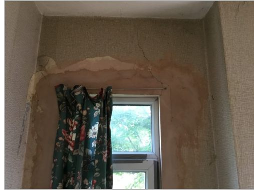
Photo - 61 Cracking in middle bedroom likely due to absence of lintel
