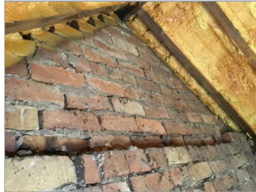
Photo - 42 Upper section of party wall is probably single skin
