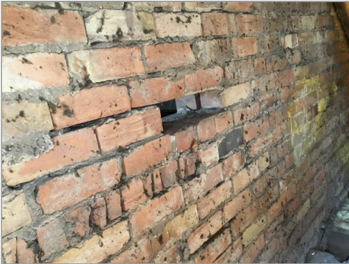
Photo - 41 Fill gap in part wall for fire safety
