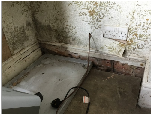
Photo - 82 Rotten skirtings in front reception
