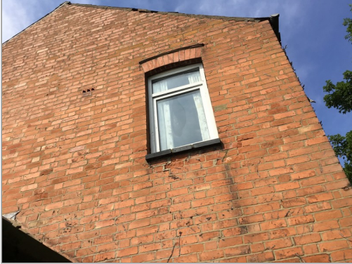
Photo - 22 Cracking to rear elevation
