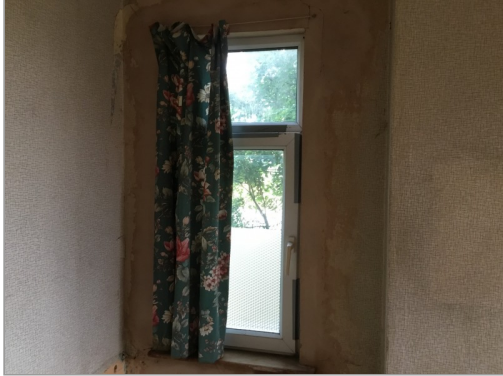
Photo - 28 Unable to open fire escape window in middle bedroom
