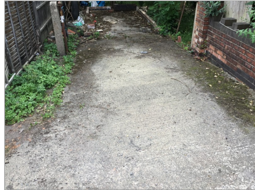
Photo - 107 Driveway cracked and in poor condition
