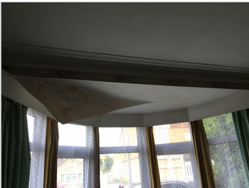
Photo - 51 Water damage to bay ceiling
