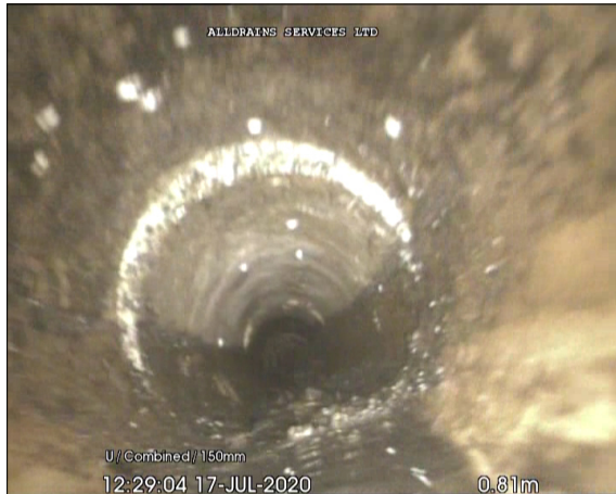
Photo: 2_4A, 00:00:09 0.91m, Joint displaced, medium (between 1.0 and 1.5 times the pipe wall thickness)
