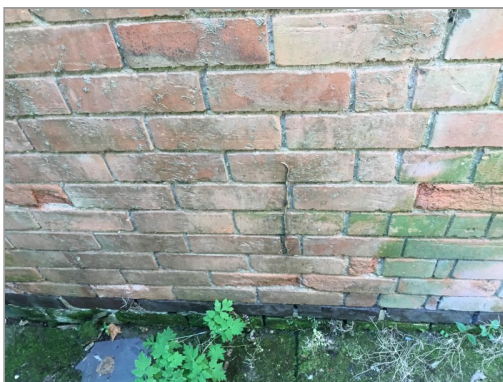
Photo - 104 Spalled and weathered bricks
