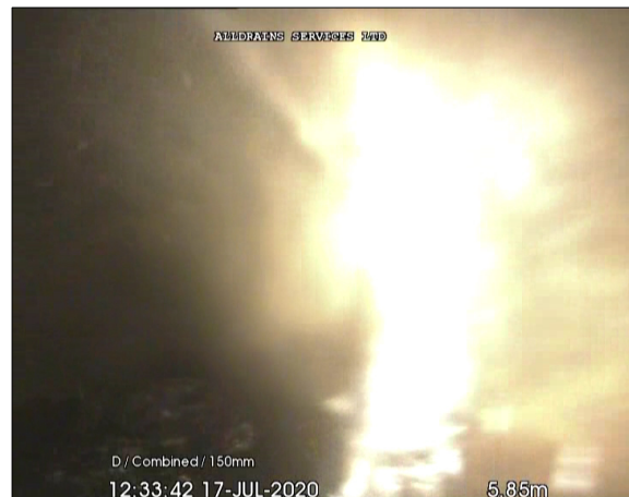
Photo: 4_8A, 00:00:41 5.68m, Joint displaced, medium (between 1.0 and 1.5 times the pipe wall thickness)
