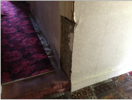
Photo - 56 Section of doorframe missing and wall repaired beneath
