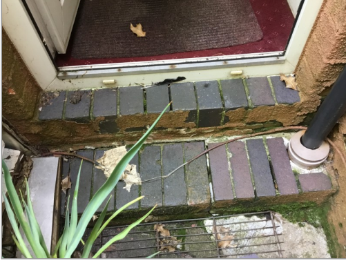
Photo - 36 Loose steps to side door
