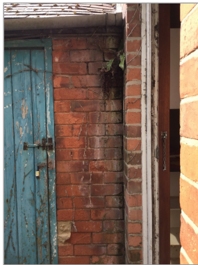
Photo - 100 Spalled and stained bricks from leaking gutter
