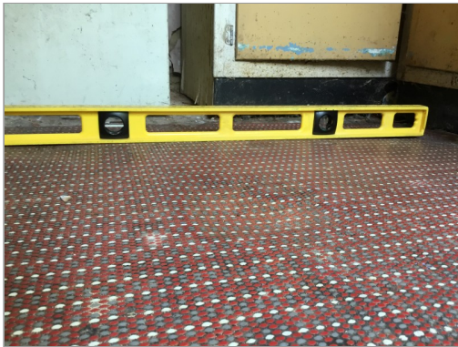
Photo - 71 Quarry tiled kitchen floor also slopes toward left elevation
